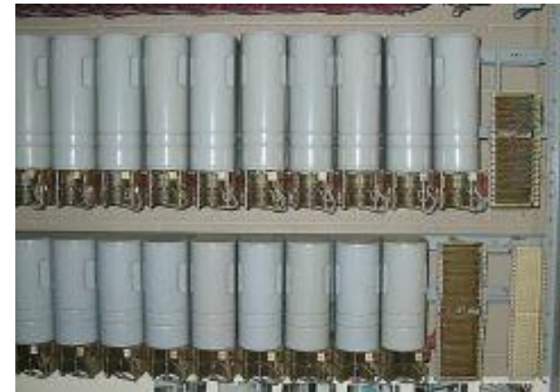
Western Electric Step by Step Community Dial Office (CDO) Quelle: phworld.org
